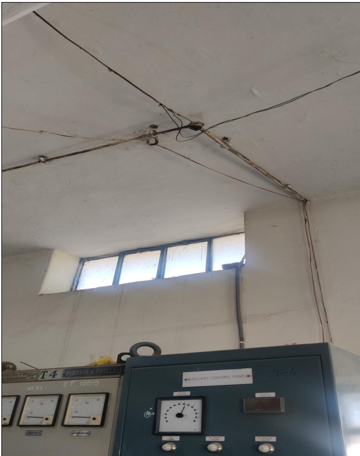
Pic 7 – Loose and hanging wires - non-compliance with NEPRA PSC section 7.46 (Fire Prevention) and Building Code Section 4.2.2 on electrical fire safety.
